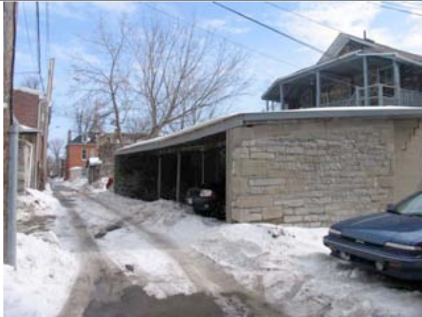
Stone 'tail' and surviving stone side wall of carriage house from lane
