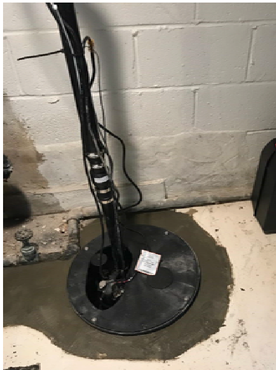
Figure 2 – Installed Sump Pump
