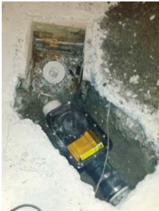
Figure 1 – Installed Backwater Valve
