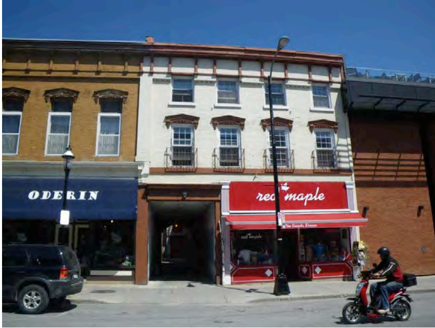
Fig.5: Carriageway at Brock St. west of King St. Note flat arch at street face semi-circular arch at courtyard.
