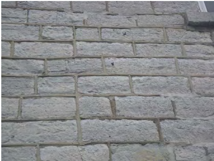
Detail: Coursing anomaly at façade of 23 Queen Street (D5)
