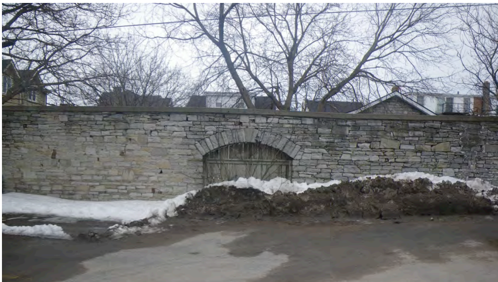
Fig.12: Wooden carriage gate at stone wall, Barrack St. west of Wellington St.
