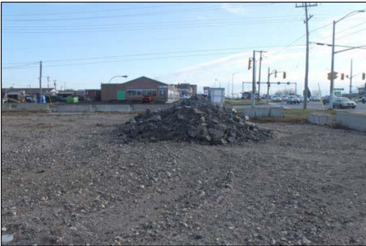
Image 6. A view of the gravel and asphalt mounded in the southeastern corner of the property.
