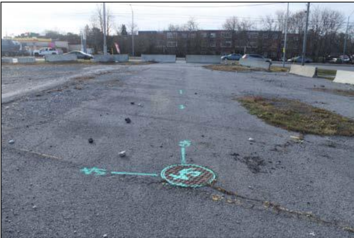
Image 4. A view of the storm sewer service line which crosses the property.
