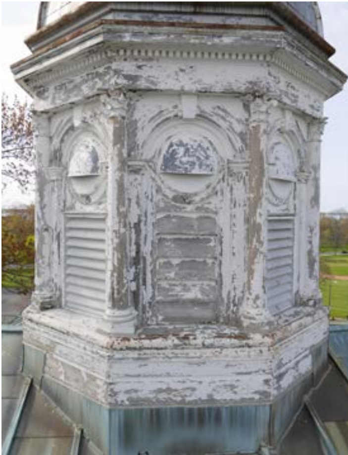
Fig. 28 East cupola. Typical loss of paint and damage of the exposed wood (THA 2017).
