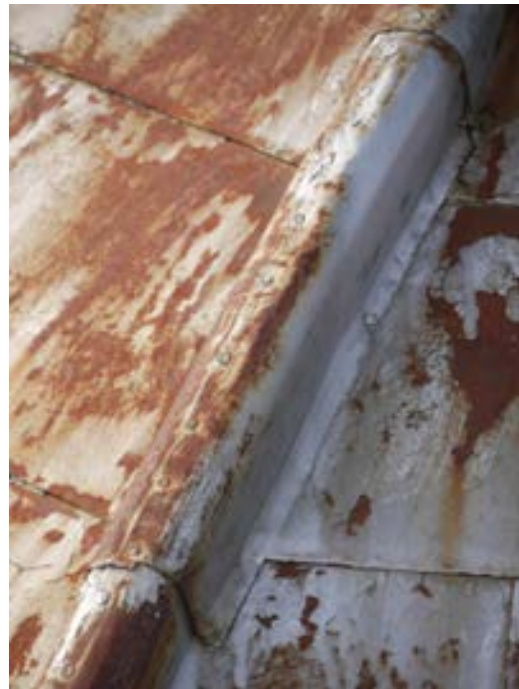
Fig. 24 East cupola. A typical ridge batten detail that appears to be functioning well (THA 2017).
