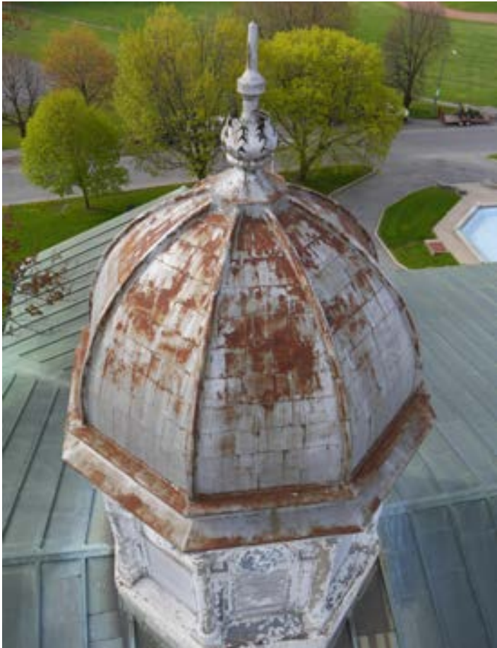
Fig. 22 East cupola. Though the zinc coated metal has reached the end of its life cycle no perforations were found in the metal. The option of repainting is available (THA 2017).
