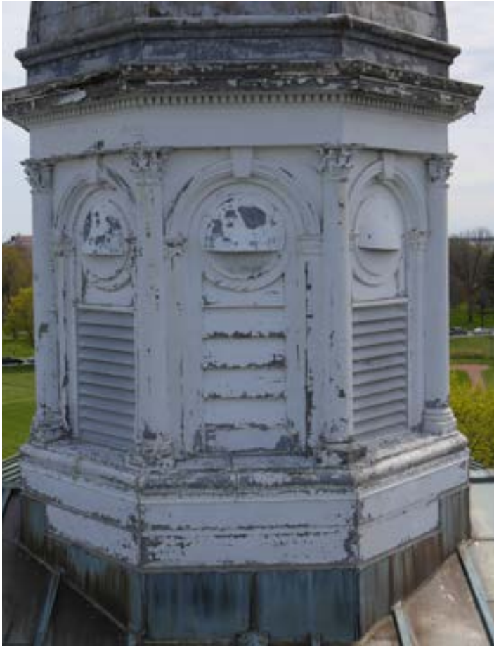
Fig. 32 West cupola. Wood detailing is in poor condition due to the higher level of exposure to south west wind, rain and sun (THA 2017).
