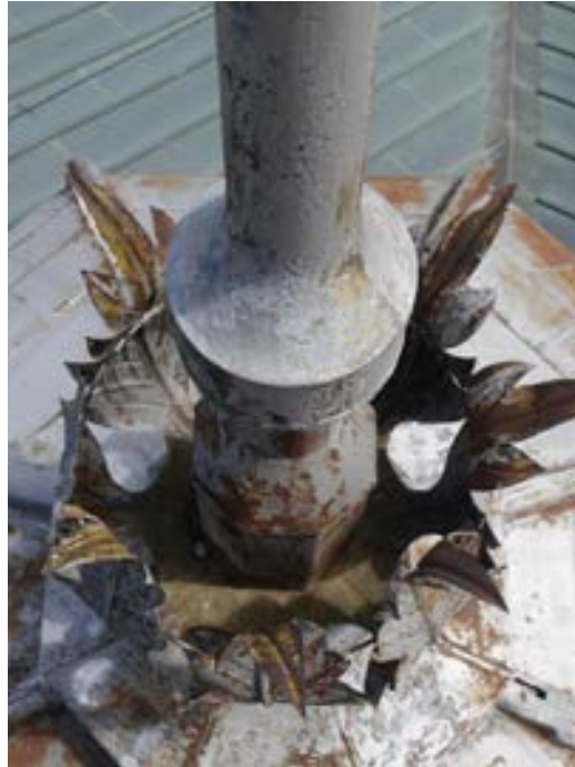
Fig. 26 West cupola. Selected finial vent cap leaves will require replacement (THA 2017).
