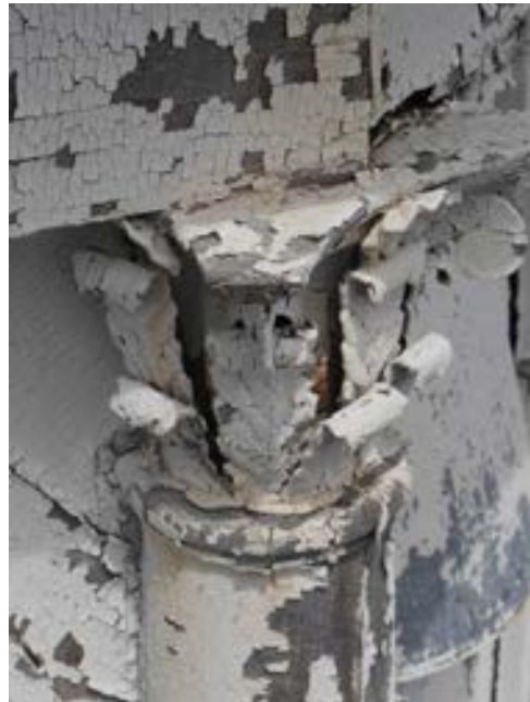
Fig. 35 West cupola. Example of loose, missing and damaged metal detailing at Corinthian capital (THA 2017).
