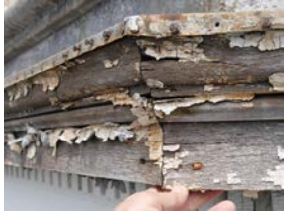
Fig. 33 West cupola. Typical example of advanced wood deterioration (THA 2017).
