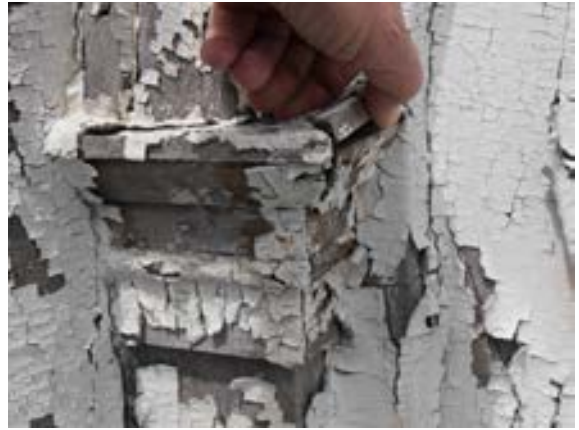
Fig. 34 West cupola. Typical example of decayed wood deterioration (THA 2017).
