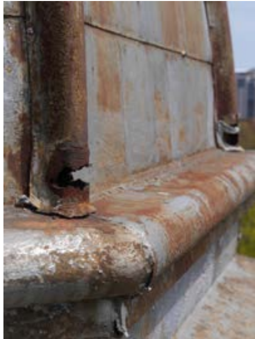
Fig. 27 West cupola. Detail of perforations in zinc coated metal and thinning of the sheet metal (THA 2017).
