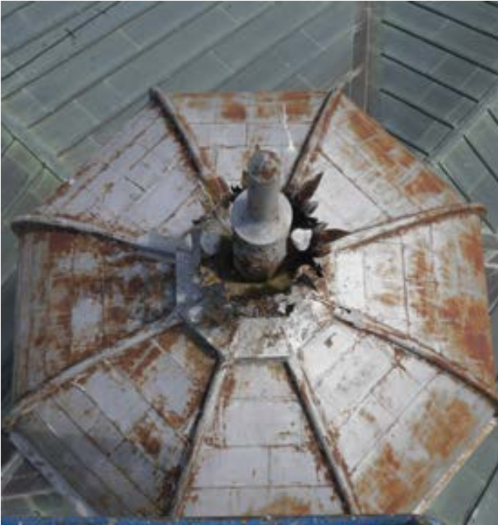
Fig. 25 West cupola. Vent cap and decorative leaves could be salvaged otherwise the life cycle of the metal roof and components has come to an end (THA 2017).
