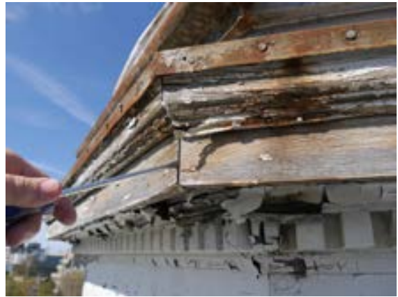
Fig. 29 East cupola. Typical decayed wood and poorly detailed drip flashing (THA 2017).
