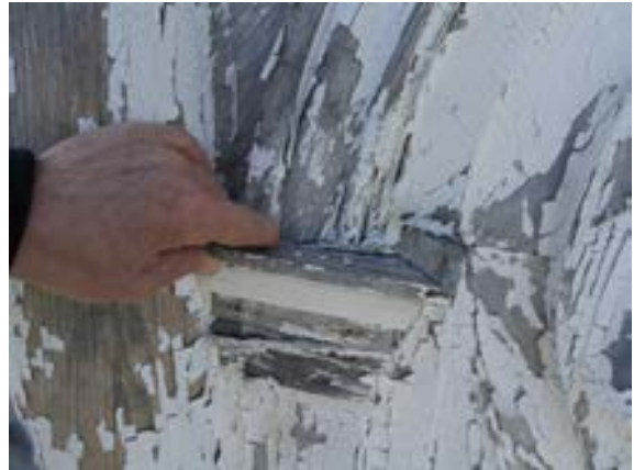
Fig. 30 East cupola. Typical example of detached decorative wood details (THA 2017).
