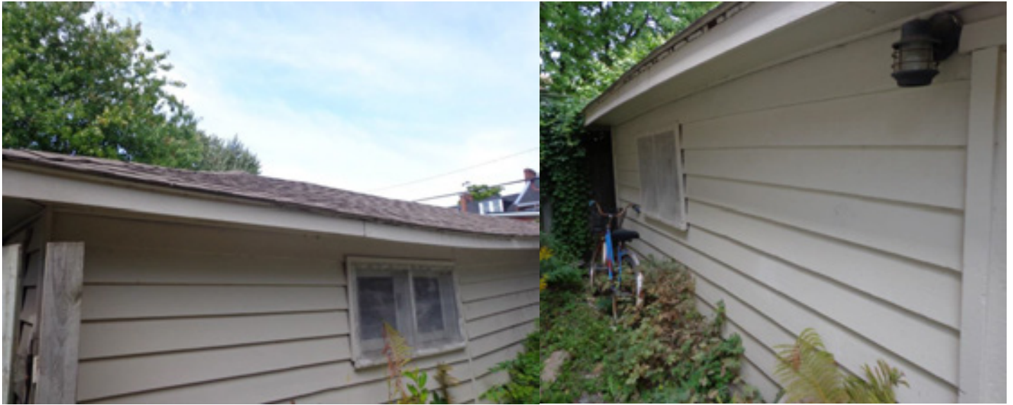
Figure 4 and 5: (Left) Roof of garage, appears structurally unsound. (Right) South façade facing rear of house.
