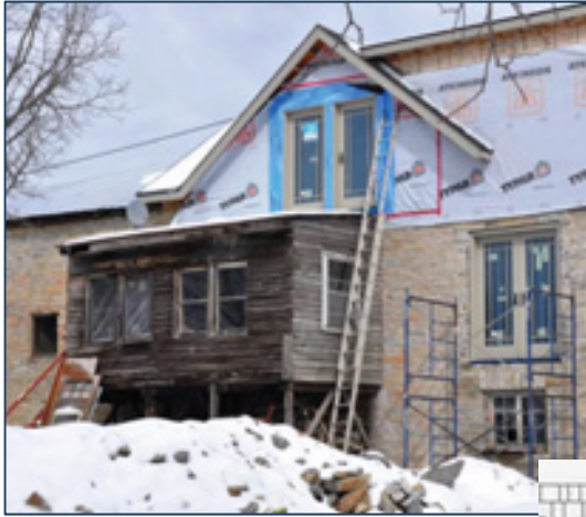
Left, existing rear addition next to the drive shed; the former has no significant heritage value and can be removed.
