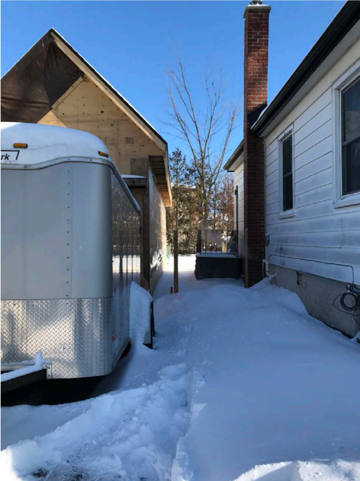
Figure 3: Existing eaves encroachment.
