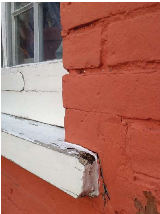
Deteriorating Window Sill
