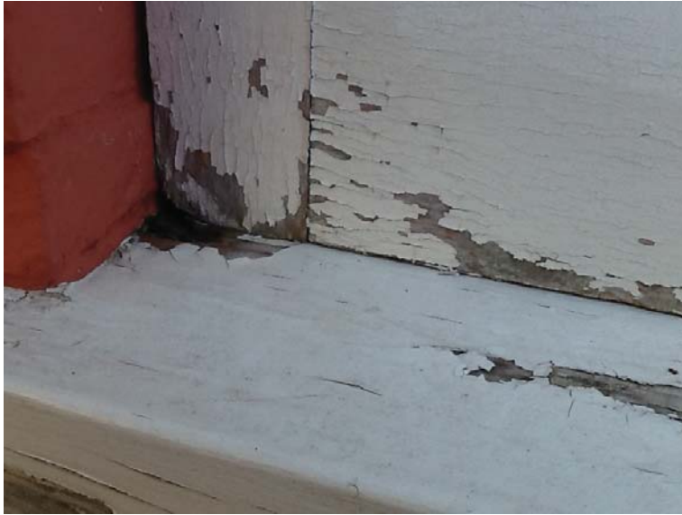
Deteriorating Window Sill
