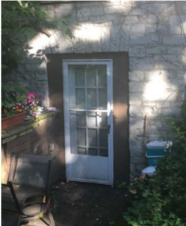
Suite - to be replaced with matching door (metal-clad wood) painted grey or black
