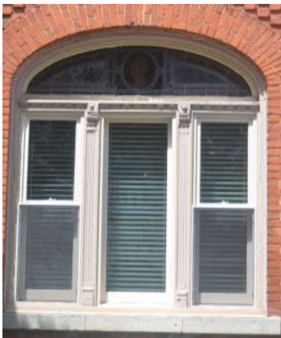
Photo A-12: 244-1 King St. E., Window Sills and Trim
