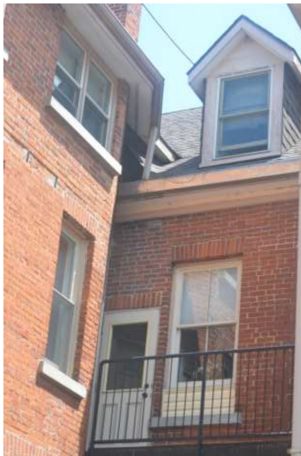
Photo A-20: 4-250 and 7-270 King St. E. Rear. Typical soffit, windows, window and door trim and gable.
