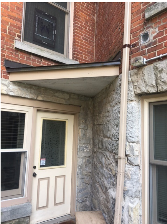
Figure 2: Photo of Roof over Back Door at 252 King St. E
