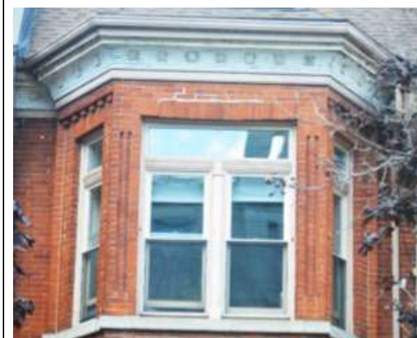
Photo A-3: 250-7 King St. E., Bay Fascia, Windows and Window Trim. 250-6 King St. E. is the same.
