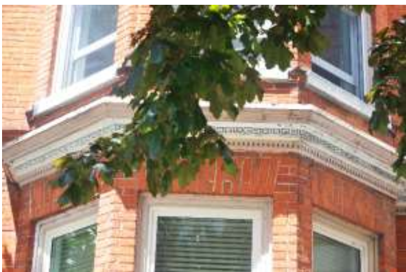
Photo A-11: 244-1 King St. E., Fascia over Bay.
