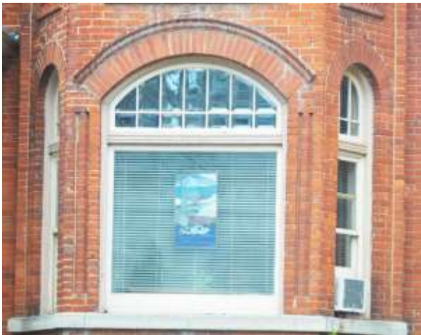
Photo A-5: 252 King St. E., Bay Windows and Window Trim. 250-1 King St. E. is the same.
