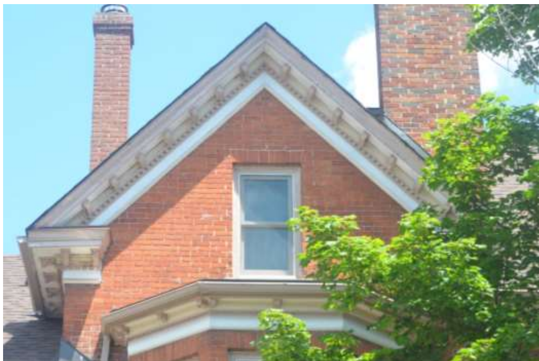
Photo A-15: 41-2 William St. Soffit and Fascia in Gable and over Bay
