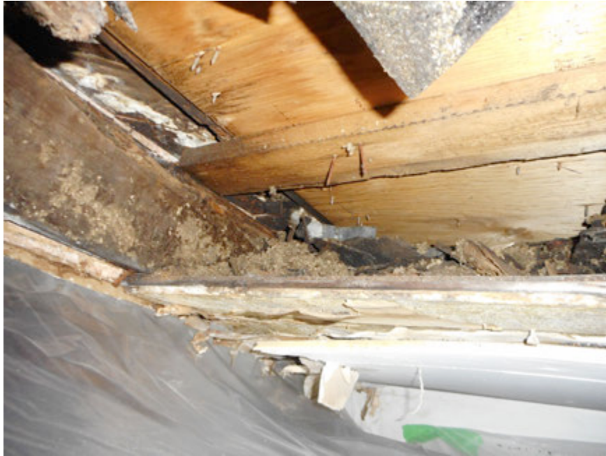
Fig.7: Serious decay and attempted past repairs at dormer. Note fungi at left.
