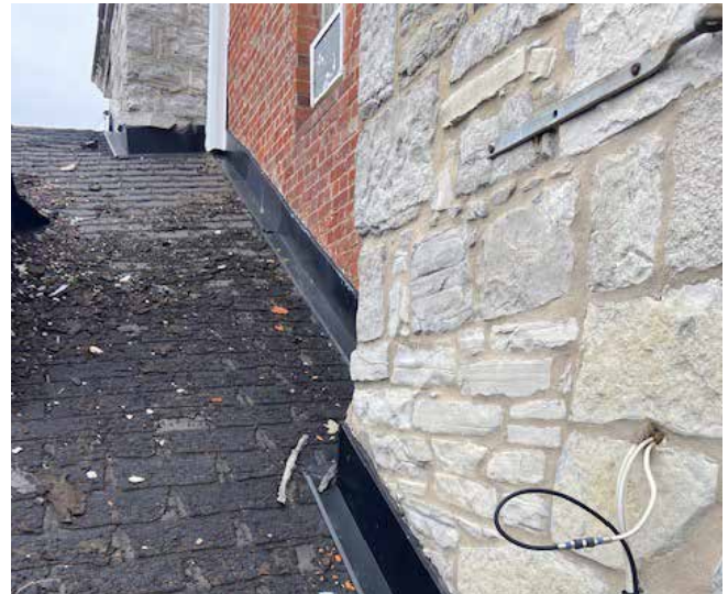
Figure 2. Shows no parapet on rear slope of existing roof on west wall.
