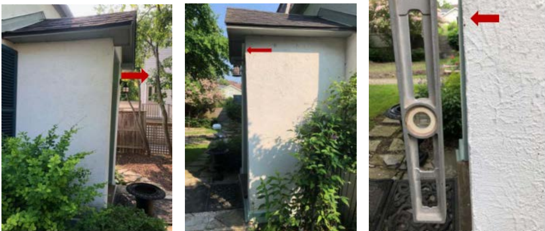
The images above show the street-facing wall four inches out of plumb. Its top leans toward the street. This is likely due to lack of a proper foundation.
