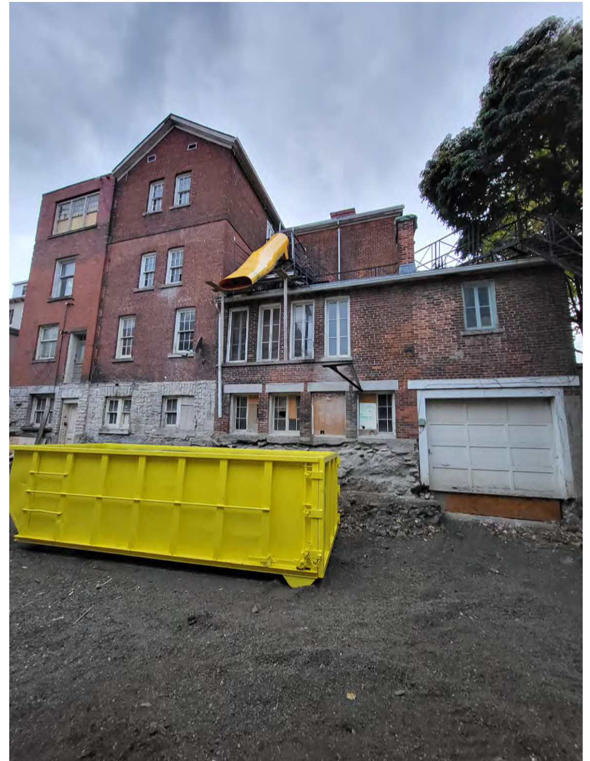
The Belvedere - Courtyard and Carriage House - Chimney to be removed 01 of 04 Shoalts and Zaback Architects Ltd. sza 22108-2_CourtyardCarriageHouse-ExPhotos_01 2024-01-22
