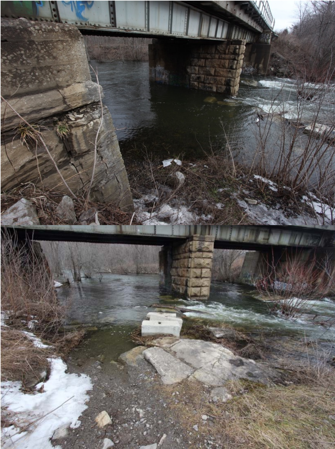
Images of Collins Creek at the CN bridge. Note that the cement blocks nearest the proposed development are submerged. These water levels are typical in Spring and Fall when fish spawning takes place. March 12, 2016.
